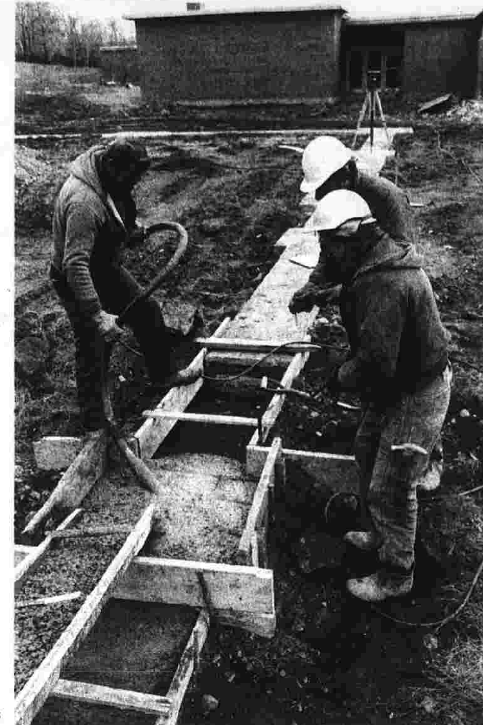
Illing Work Goes On Despite Cold Cold weather does not deter construction at Illing Junior High School as Robert Porter, left, John Rodrigues, center, and partner of the B&R Construction Co. and Larry Cyr work together to pour concrete footings for the interior walls of the new gymnasium. (Herald photo by Dunn)
